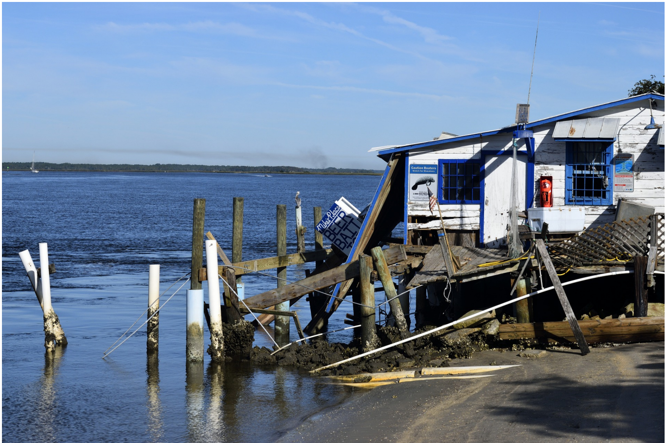
Damage from Hurricane Matthew
